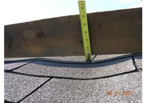
Example of collapsing roof sheathing due to moisture induced wood rot above a cathedral style ceiling.
